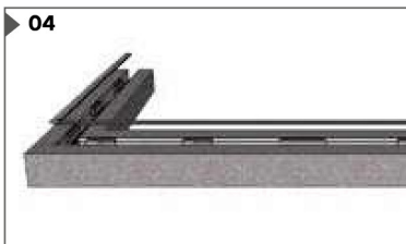
Fixed the outside system cover on the outer face of the blocks.
